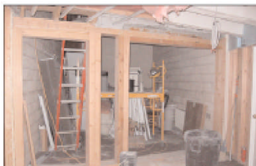
With the CMU wall gone, framing is in place to accommodate a spiral staircase and double doors to the piano storage room.
